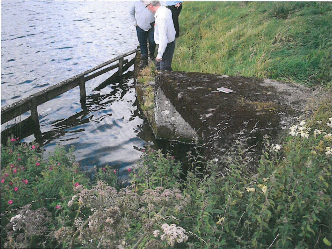
Photo 6 – Spillway inlet showing damaged baffle board
